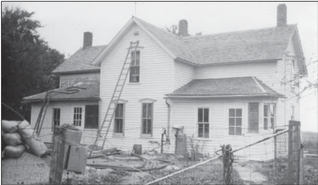
The house where Rosa and David Dady lived. Rosa added the left section after David's death in 1916. Fred Baade and family lived in the house and farmed the Dady farm from the late 1920s until Helen and her family moved there in 1945 when this photo of renovating and blowing insulation into the walls of the place was taken. North side, Section 13, Roosevelt Township. The house was moved when a new one was built in 1956. The Deane and Marion Gunderson collection.
